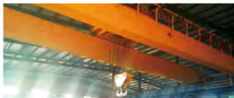
起重设备 载重量100t, 32t, 20t, 10t Hoisting Equipment Load Capacity 100t, 32t, 20t, 10t
